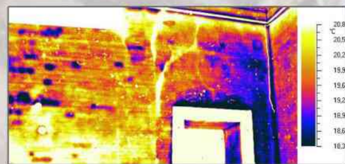
Fig. 5, IR Thermograms composite of wall "B", room # 5
