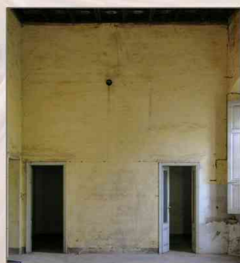
Fig. 7, visual state of wall "B", room n 9
