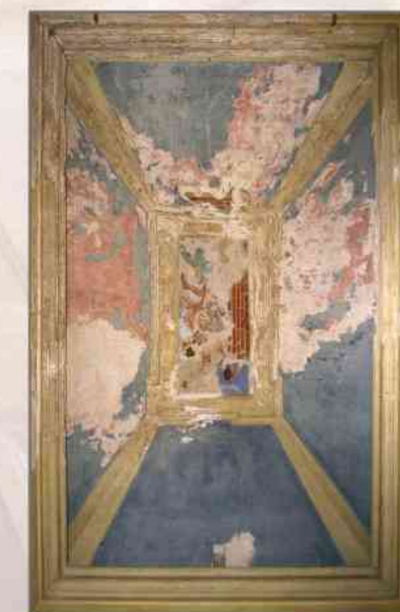
Fig. 9, visual state of vault in room # 6; damage of surface (stains, lack of color, lack of plaster, etc) masks delamination.
